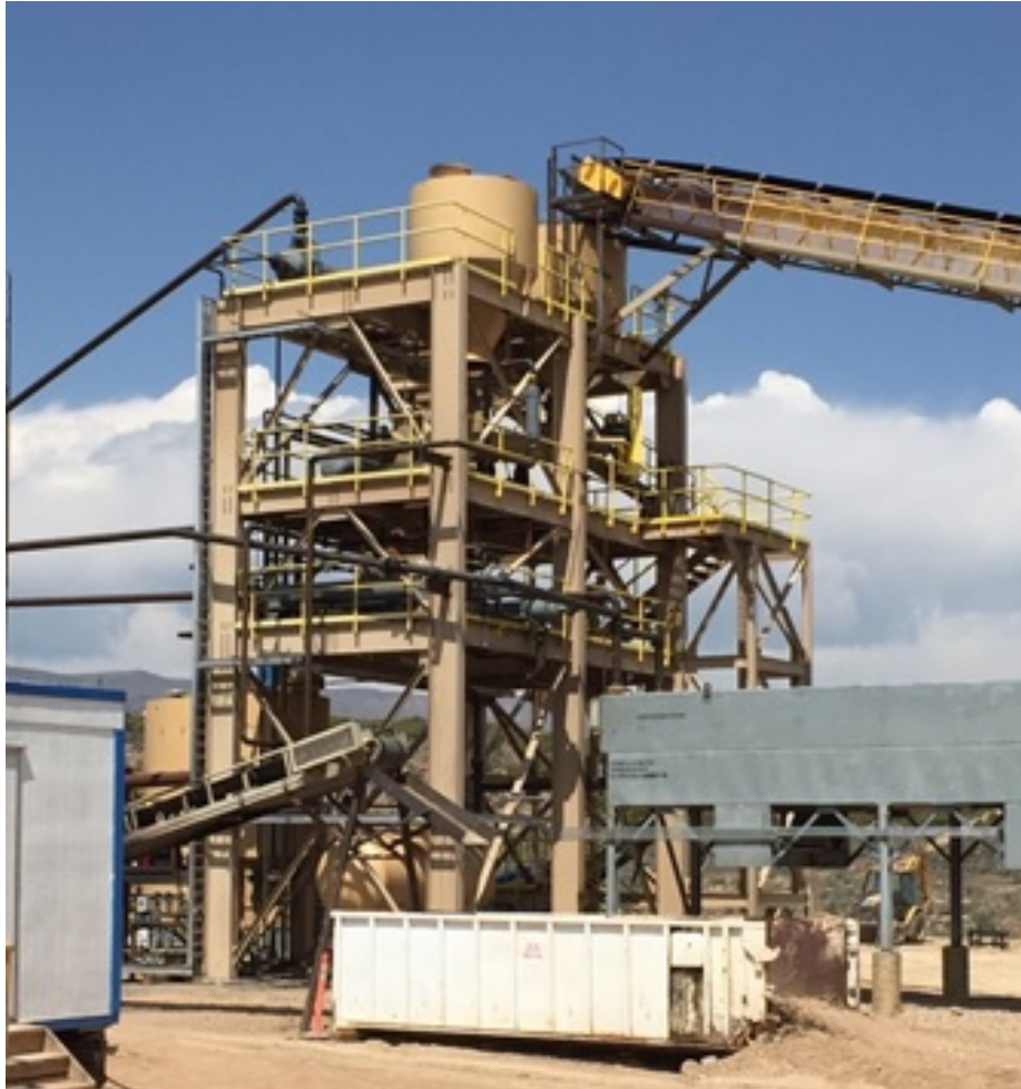
Figure 1. Conveyor belt loading oil sands ore into the premixing vessel at the top of MCW's oil sands extraction facility in Maeser, Utah, USA. The gray, horizontal structure immediately below the conveyor belt is the chiller used to condense all the vaporized solvent that is collected from the sand drying vessel. The condensed solvent is recycled through the closed loop system and reused.
