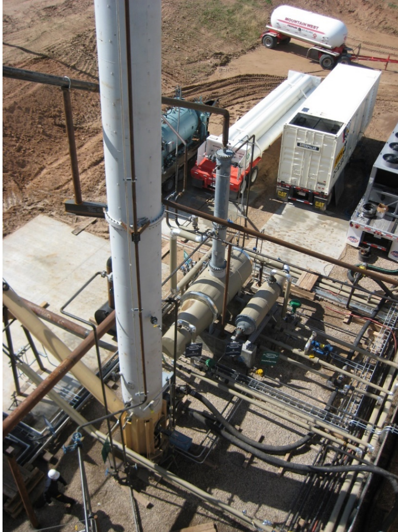
Figure 2. MCW patented, pseudo-boiling fluidized bed extraction column in the foreground. The extraction column increases oil recovery to over 99%. The distillation column used for separating the solvent from the oil is in the background. All vaporized solvent is collected, condensed (see chiller in figure 1) and recycled in the closed loop system.
